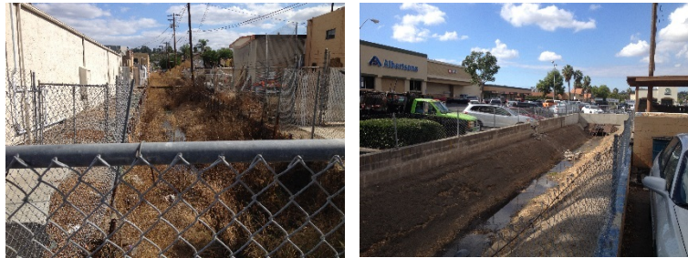
Photos of alley storm drainage channel and undersized pipe
